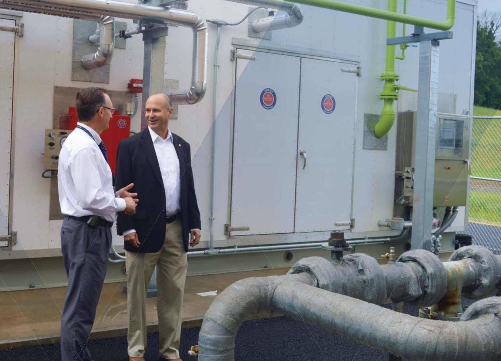
Milton S. Hershey Medical Center Campus Energy Engineer Kevin Kanoff (left) and UGI's Steve Bareuther (right) tour the Center's new CHP plant.
